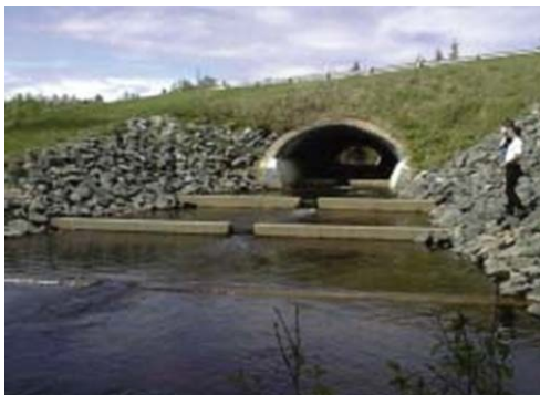
Figure 23. Concrete weirs are used as control structures in a watercourse to raise the downstream water elevation at a retrofitted culvert.
